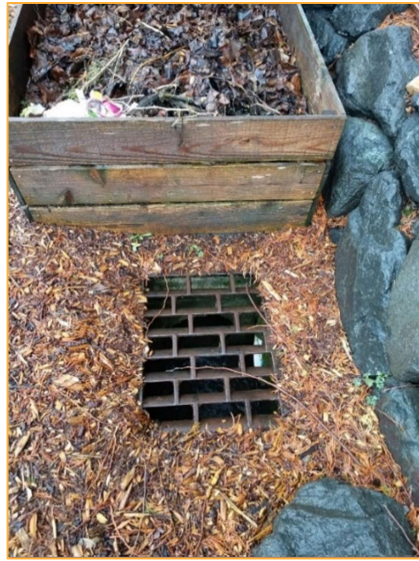
Photo S9 – Facing west along the north side of SE 30 th St approximately 65 feet west of Photo S8. Runoff is conveyed west toward Lake Washington.
