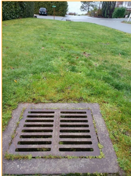
Photo N8 – Facing west along SE 28 th St approximately 40 feet west of Photo N7. Runoff is conveyed via this catch basin on the south side of the street toward Lake Washington.
