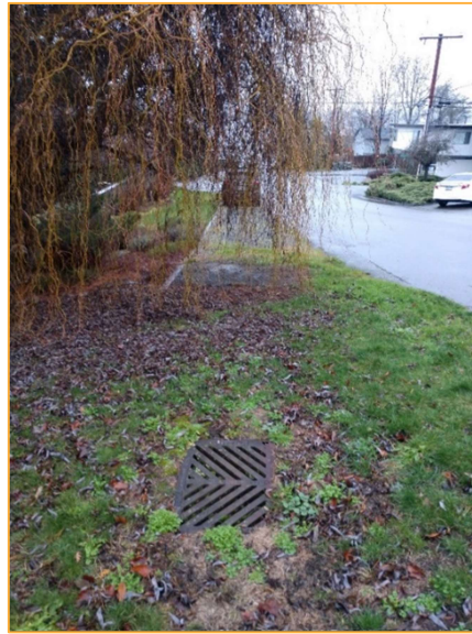
Photo N5 – Facing west along SE 28 th St approximately 95 feet west of Photo N4. Runoff is conveyed via this catch basin on the south side of the street toward Lake Washington.
